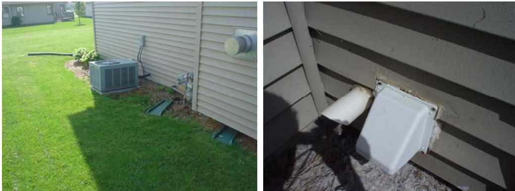
Negative grade - Caulk around dryer vent
