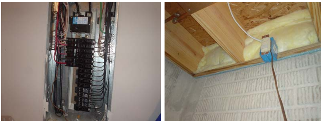
Main Panel View - Extension cord wiring
